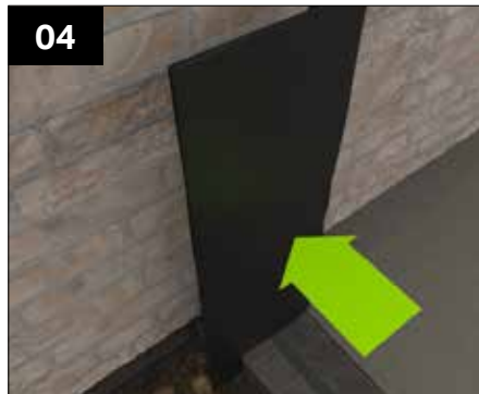
04 Insert the DPC into the channel created, this will require folding into an 'L' shape, the DPC may require cutting to seat correctly. Use packers to keep the DPC in place. Once the walling panels are fitted this will then be folded again to form a 'Z' shape. If required repeat this and the previous two steps on other junctions with the existing structure.
